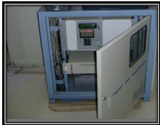
Fig. 1.7 Installation of Front End Processor
