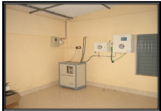
Fig. 1.6 Intelligent Electronic Device installation
