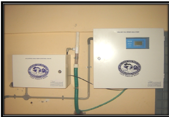
Fig. 1.4 Chlorine analyzer installation
